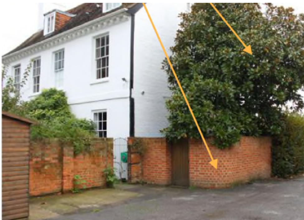
Figure 4. Shows the original southern wall (left of the photograph) – buttressed and Flemish Bond. Note, the contemporary wall to the right copies the style, but is obviously modern.
